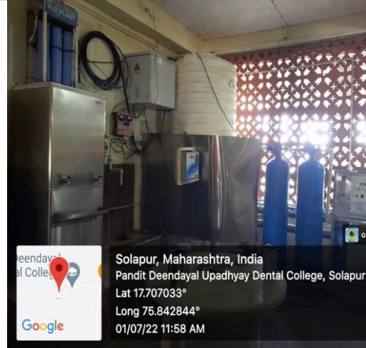
Water purification plant
